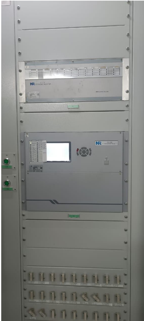
Lampiran A.2 Nameplate Generator Transformer Unit 3 PLTU Pangkalan Susu
